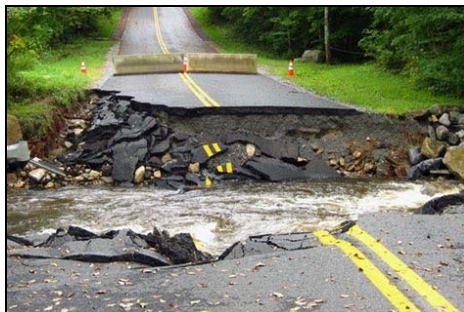
Washout From Undersize Culvert
